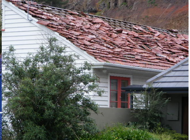
Should have wired down the roof tiles
